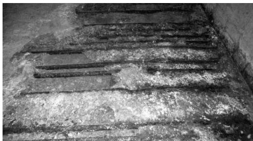
Damage in ventilation tubes, 2015
