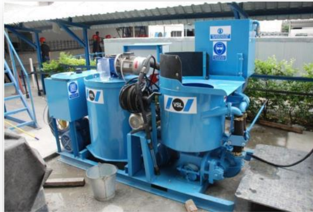
VSL grout mixer
