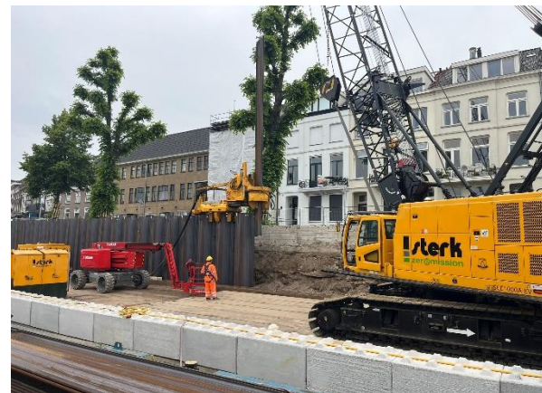
Silentpiller 250kW Retrofit + Sany SCE1000EV
